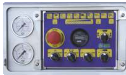
Panou de control electromecanic
